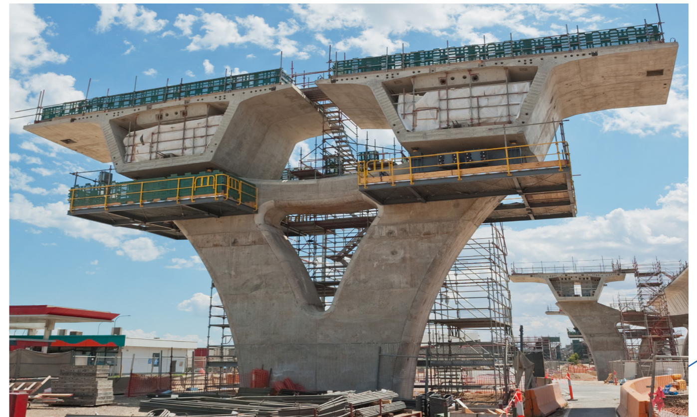
Traffic Management along Cornish Street during the construction of Infinity bridge double deck.
